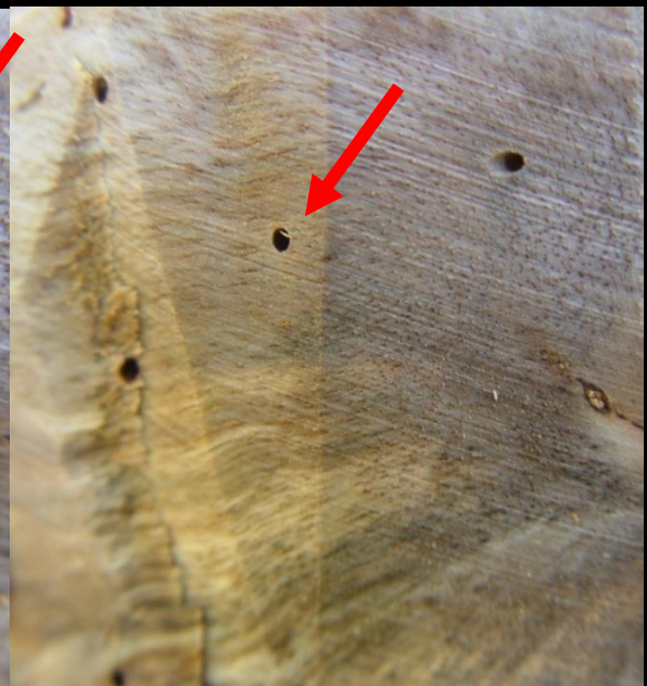
Perforation by borers
