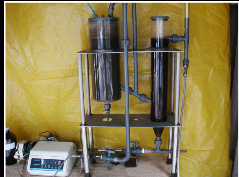
Activated sludge plant
